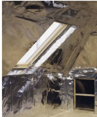
Thermo-Foil ES being installed in an attic room prior to fitting plasterboard
