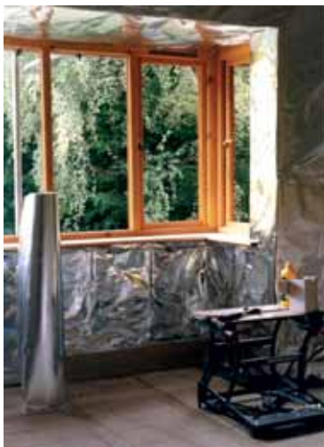
Apollo HPA adhesive tape being used to seal a Heat Reflecting Membrane installed in a private home prior to fitting plasterboard
