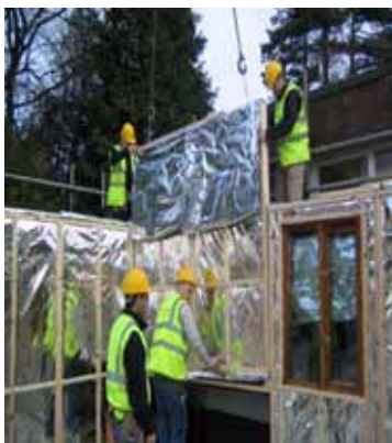
Eco-Brite installed in prefabricated wall panels
