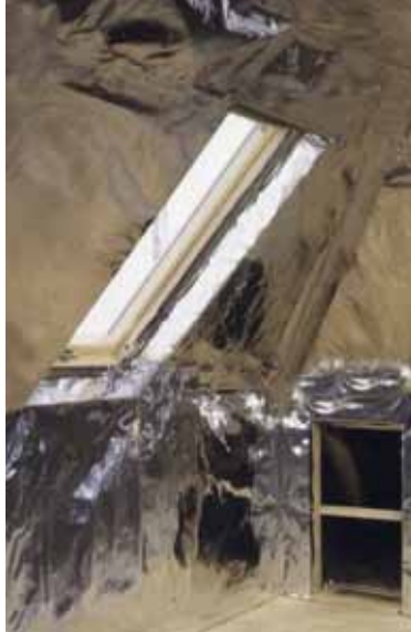
Thermo-Foil ES being installed in a private home prior to fitting plasterboard
