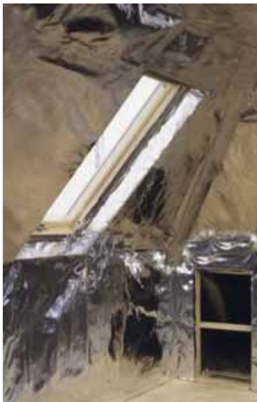
HRM I being installed in an attic room prior to fitting plasterboard
